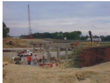
CDS will assist you to stake out pilings and foundations, and analyze design conformance
